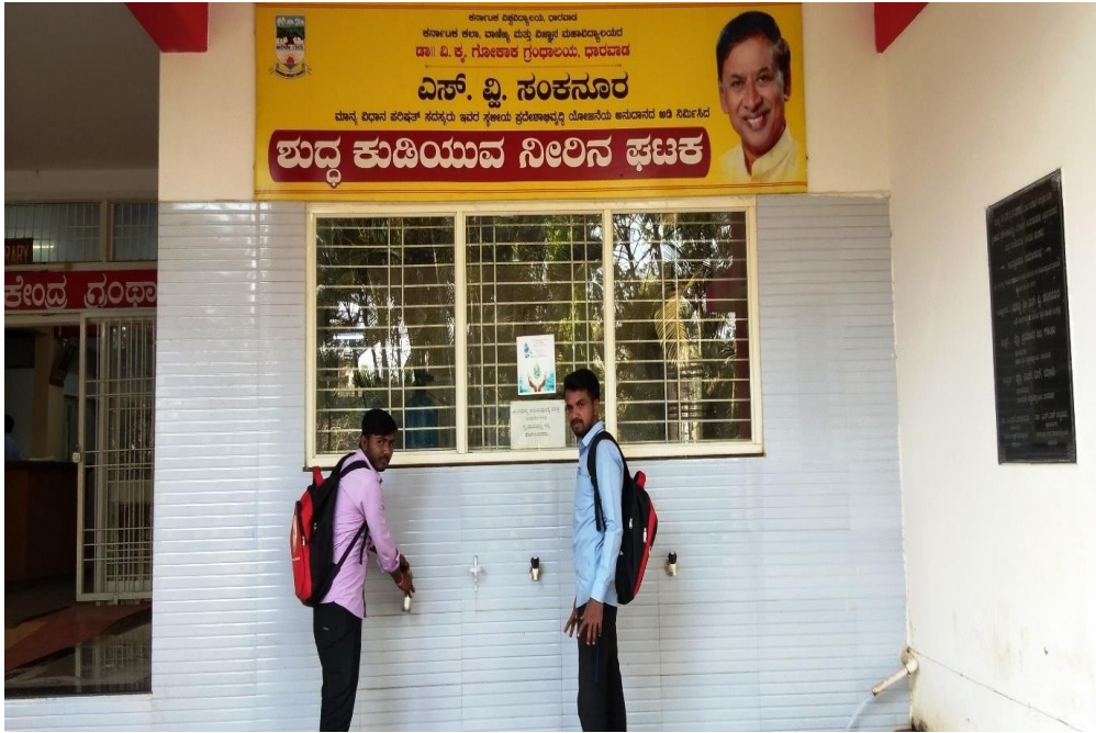
Reverse Osmosis (RO) drinking water facility for students and Staff at Dr.V.K.Gokak Library
